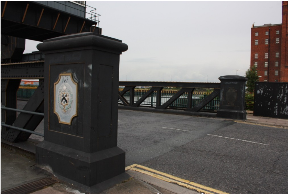
Plate 12: View of the two cast iron plinths at the west abutment of the bridge. Identical plinths are sited at the east abutment
