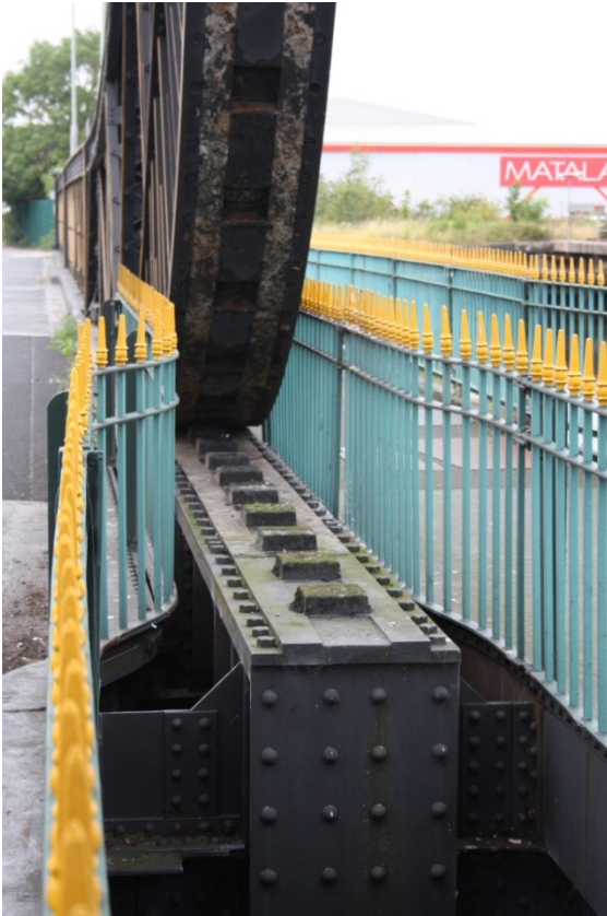
Plate 11: View of the curved and toothed rolling end of the lifting span characteristic of Scherzer rolling lift bridges
