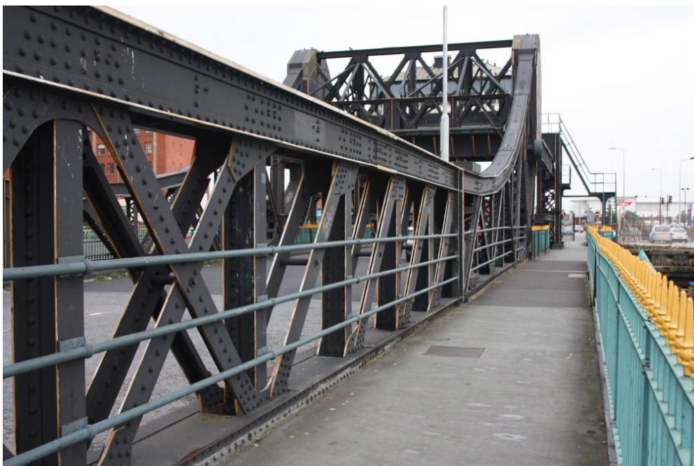
Plate 10: Close up view of lattice girder parapet, ramping up towards the lifting end
