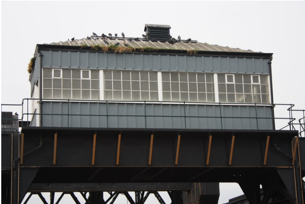
Plate 17: View of the bridge house showing wrap around windows with glazing bars, and hipped roof and asbestos sheet cladding.
