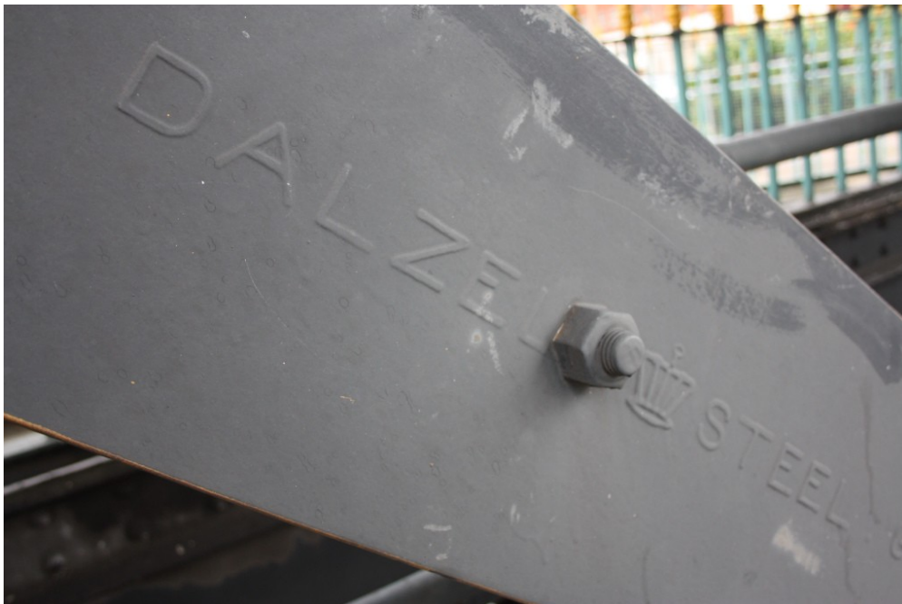
Plate 18: Example of steel member showing maker's name - in this instance Dalzel Steel
