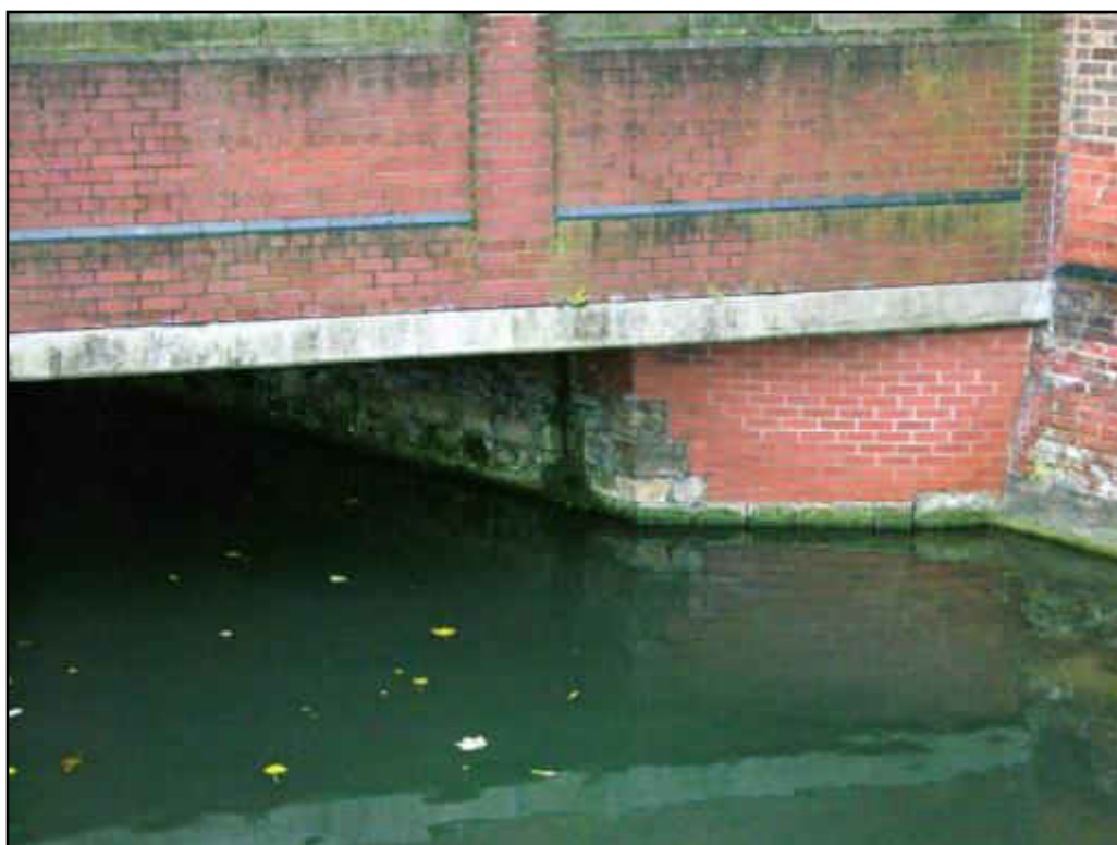
The modern Haven Bridge showing the limestone foundations of the former Stone Bridge
